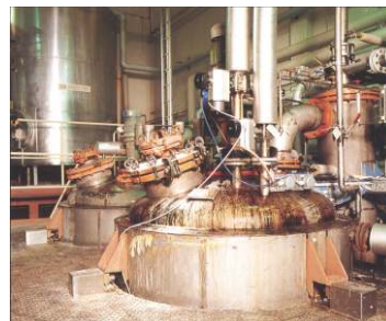
Batching Processes Reactors and Process Vessels
